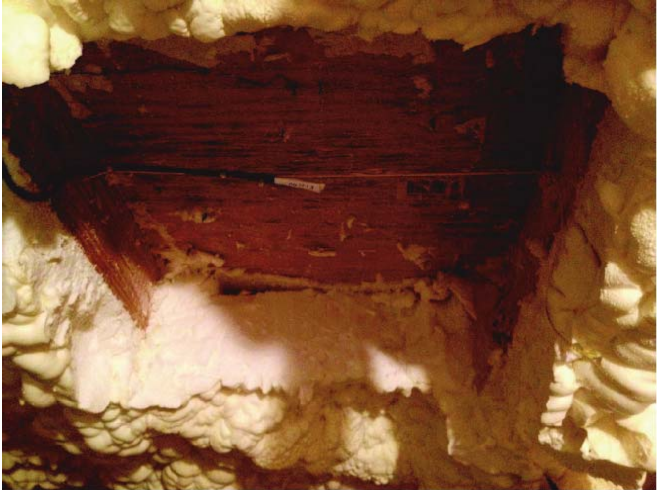
Figure 1. Taken from Miller et. al. 2016, Figure 5, showing the roof sheathing and rafters on the north-facing roof after two years of climatic exposure with ocSPF insulation removed for inspection
